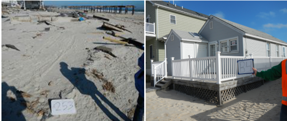
Figure 1. Contrast between large damage in an area with eroded dunes (left), and minimal damage in a more protected area with intact dunes (right).
